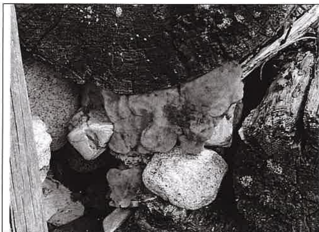
Photo 1: Urea-formaldehyde insulation within the fill of the wall
