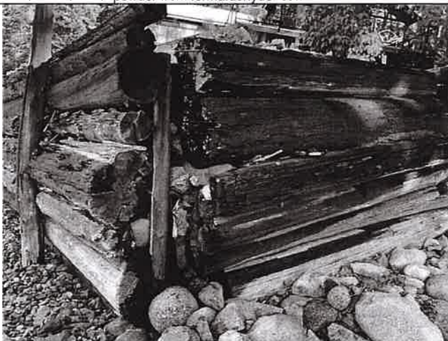
Photo 4: Close-up of bulging wall with foam and plastic debris (southwest corner)
